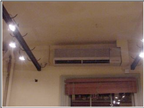
Heaters over windows
