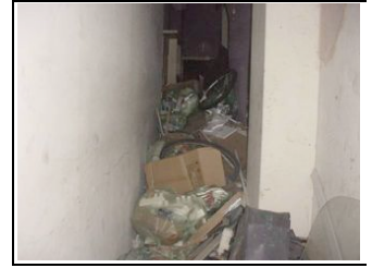
Rubbish in stair area
