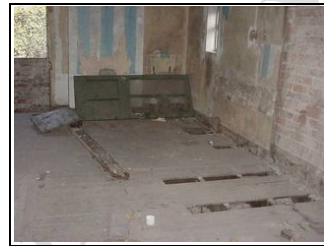
Floor sections missing
