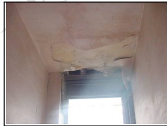
Leak above front door
