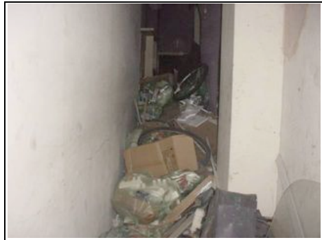
Rubbish in hallway/stairs
