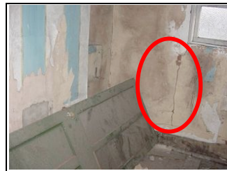
Vertical crack right approx 1m
