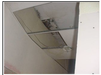
Missing ceiling tiles
