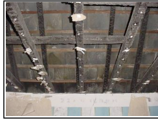
Burnt roof timbers
