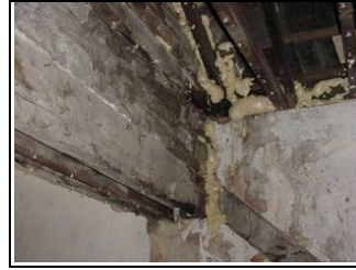
Rear area joins front area - lintel
