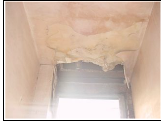
Dilapidated window and ceiling
