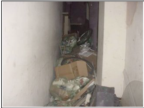
Rubbish in hallway/stairs
