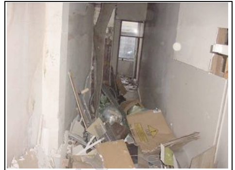
Hallway with debris
