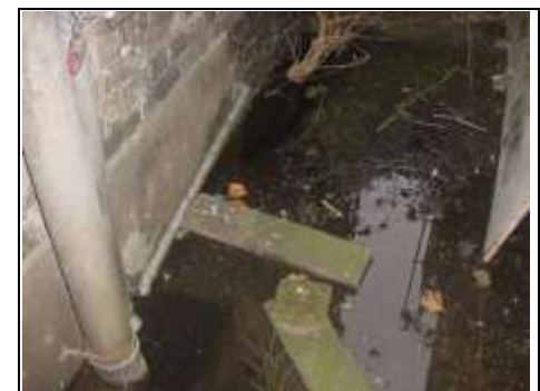
Flooding to passage way when taps had been run
