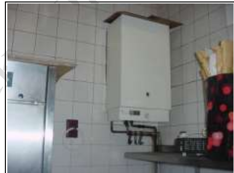
Boiler in kitchen
