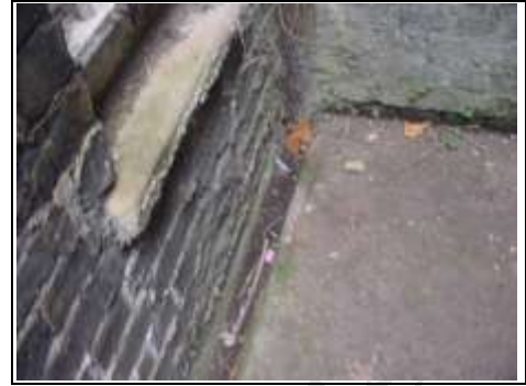
Brickwork frequently damp
