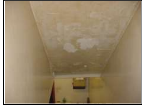
Ceiling requiring redecoration
