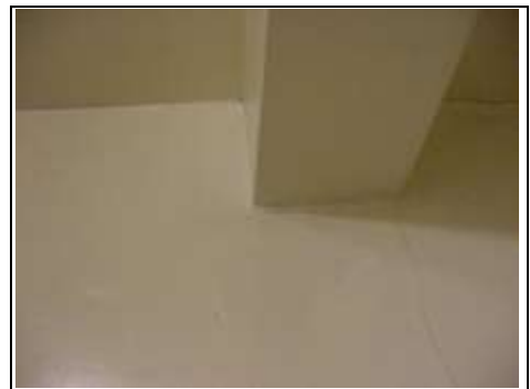
Cracking around spin beam in store
