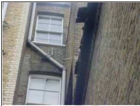
Slates hanging off
