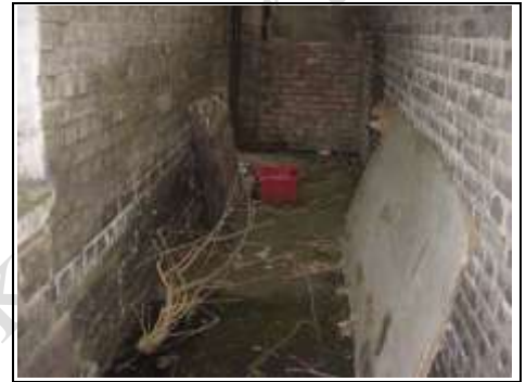
Flooding to rear property when taps had been run due to blocked drain in passage way
