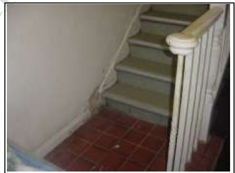
Dampness in the property
