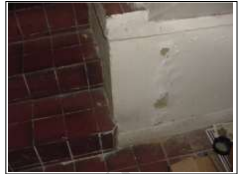
Internal dampness at basement level
