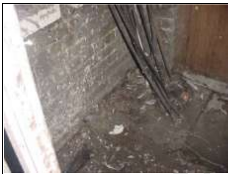
Drainage rods stored to rear are always good indicators that the drains block a lot
