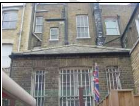
Kitchen roof disperses rainwater directly onto nursery
