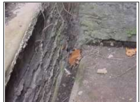
Gully around rear of the property that needs clearing
