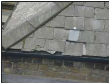
Close up of miss placed and broken slates
