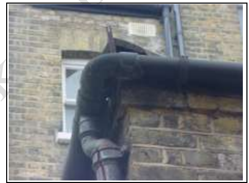
Plastic gutter and cast iron downpipe cracked
