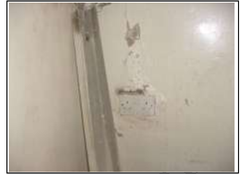
Lateral dampness on party wall
