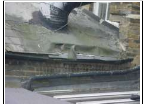
Gutter is discharging onto next door's roof
