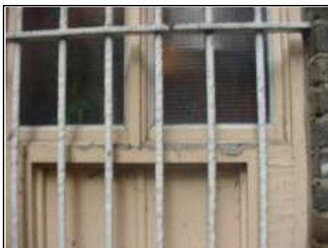
Flaky paint to window likely to require repair
