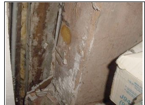
Dampness in vaults
