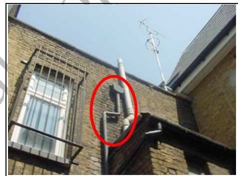
Cracking centrally to the rear
