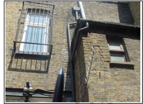
Cracking and differential movement to right side
