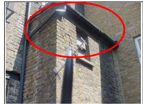
Signs of movement to rear toilet block
