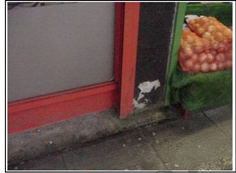
Plaster/column needs decorating
