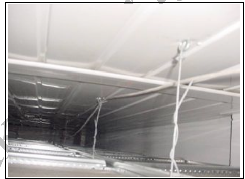
Plastic cladding above suspended ceiling
