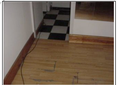
Worn floor to rear
