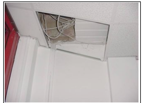
Opening in ceiling with sign of front flat roof leaking
