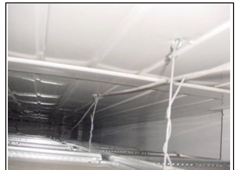
Plastic cladding above suspended ceiling
