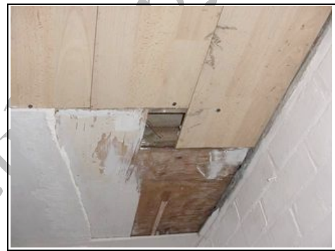
Hole in ceiling in toilet
