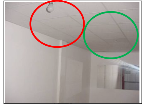
Light bulb (red circle) Hole in ceiling tile (green circle) where traditional lights rather than Category II commercial quality lights
