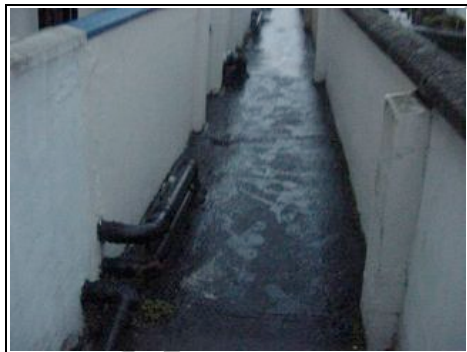
Walkway in poor condition
