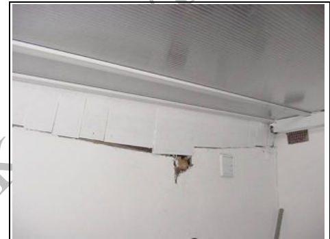
Poor infilling on conservatory
