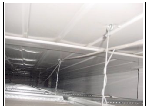
Plastic cladding above suspended ceiling 16
