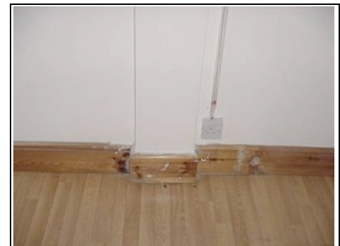
Damp to left side of property
