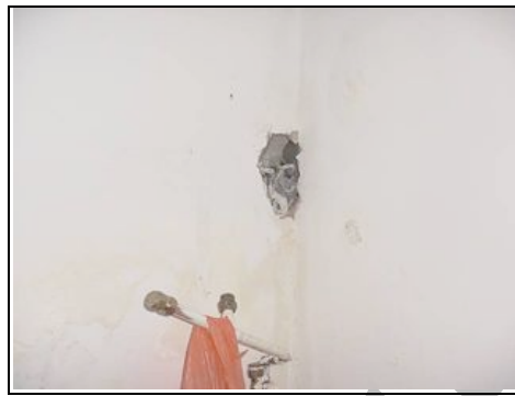
Hole in ceiling in toilet
