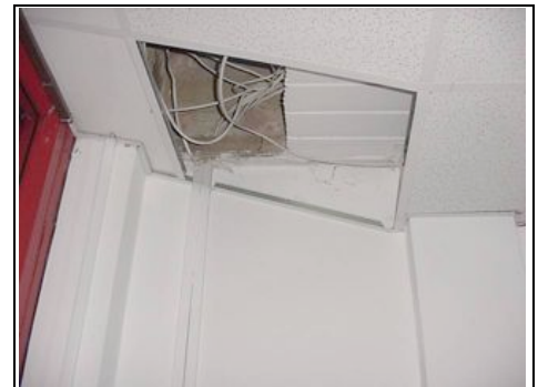
Opening in ceiling – flat roof leaking
