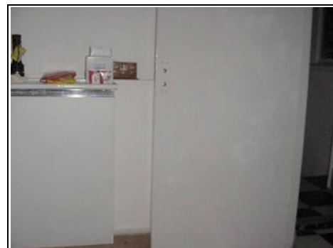
Door to office requires ironmongery
