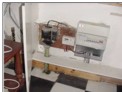
Electric fuseboard in office
